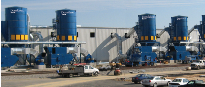
776RF at Wood Furniture Plant
