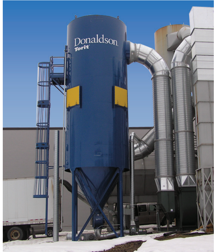
376RF at Cabinet Shop
