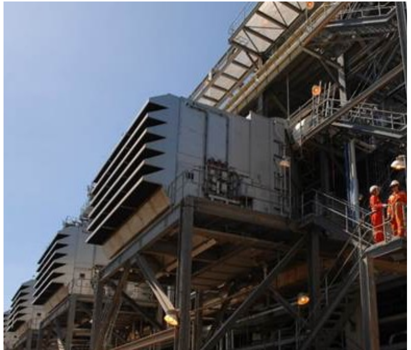
At the LNG plant, 720 pairs of Donaldson filters provide clean air to six LM2500 G4 gas turbines
