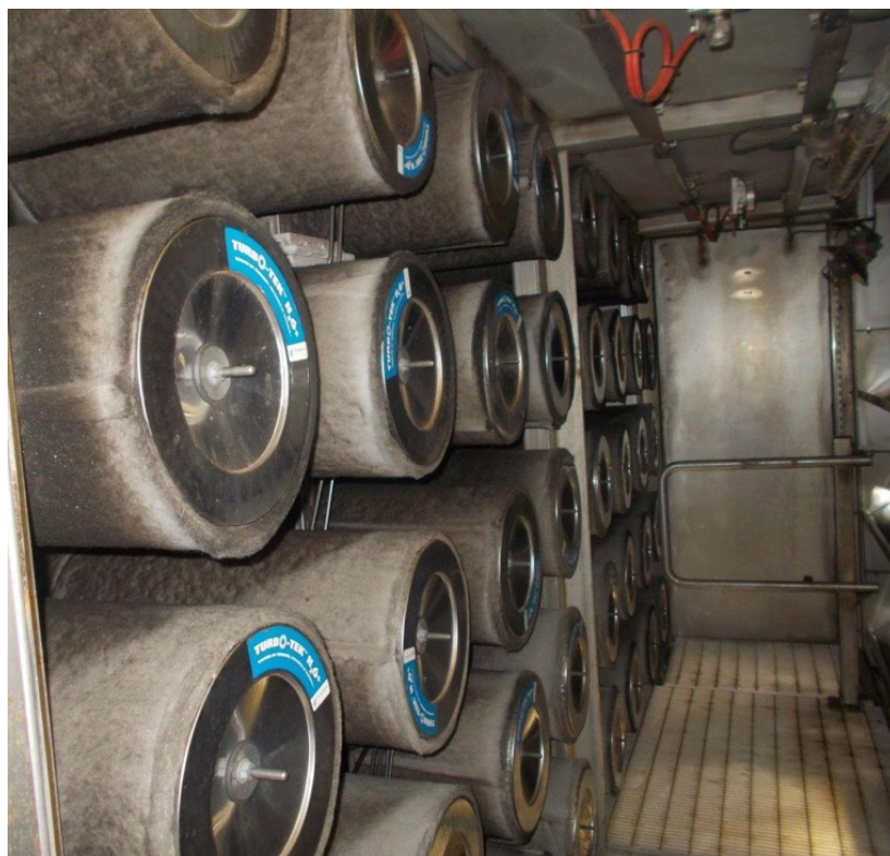
Despite bushfire soot build-up at 6,000 hours, there was little to no spike in differential pressure or blade health.
