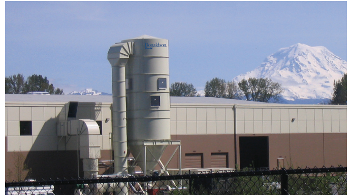
528LP12 at Cabinet Factory 70,000 cfm (118,906 m 3 /h)
