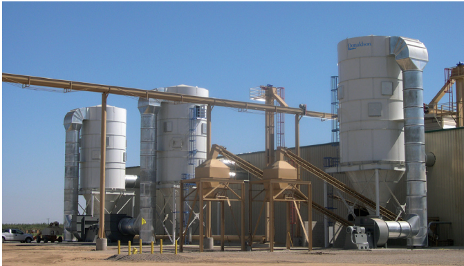
THREE 684LP12 at Almond Shelling Plant 100,000 cfm/each (169,865 m 3 /h each)
