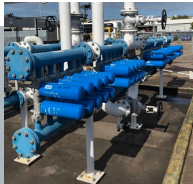
Bank of five P568933 Manifolds with fifty DBB8777 filter elements installed
